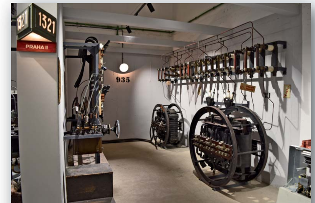
3 000 V transformer station No. 935, with dry-type transformers
